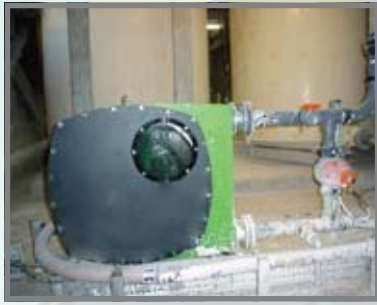
■ Water treatment - Lime mixing & recirculation
