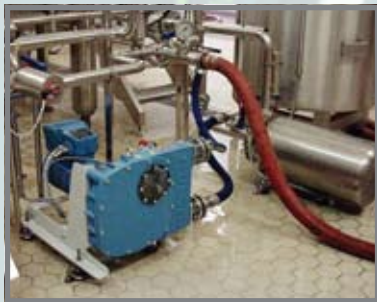
■ Brewing - Pumping Kieselguhr
